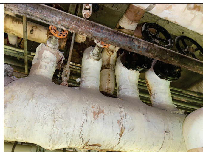
PHOTO 4 TSI-04: 4" Mudded Fittings (White) (5% Amosite and 10% Chrysotile) and non-ACM wrap.
