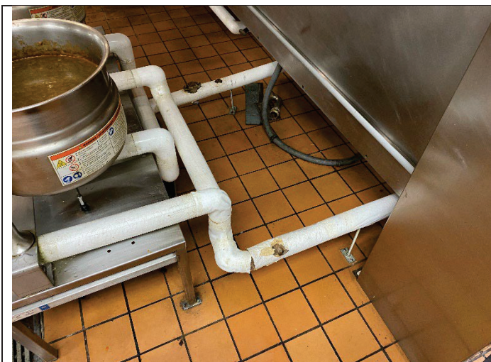
PHOTO 1 TSI-01: Fiberglass Pipe Wrap w/ Mastic (White) 2" Pipe
