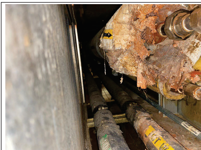
PHOTO 2 TSI-02: Fiberglass Pipe Wrap w/ Mastic (White) 4" Pipe
