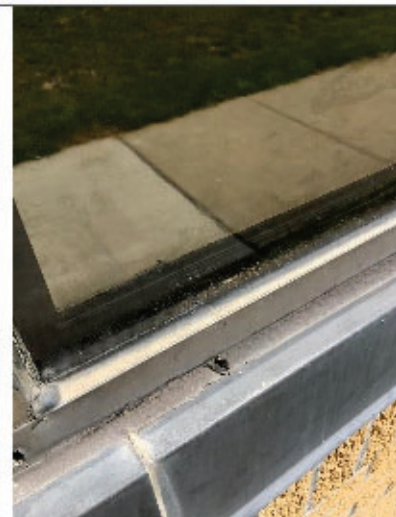
PHOTO 6 | Black Caulk Exterior Windows 3% Chrysotile
