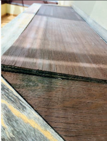
PHOTO 3 Brown Painted Shelves < 0.5% lead (by weight)
