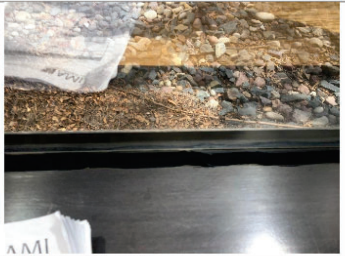
PHOTO 4 | Black Caulk Atrium Non-ACM
