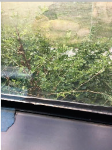
PHOTO 3 | Black Caulk Atrium Non-ACM
