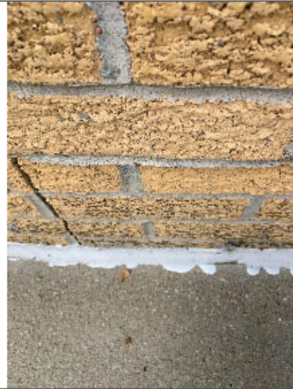
PHOTO 8 Gray Base Exterior Caulk Non-ACM
