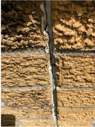
PHOTO 7 Gray Exterior Vertical Seam Caulk 5% Chrysotile
