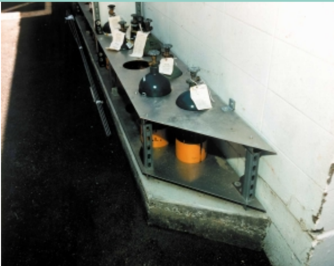
Figure 82: Small gas cylinder storage.
