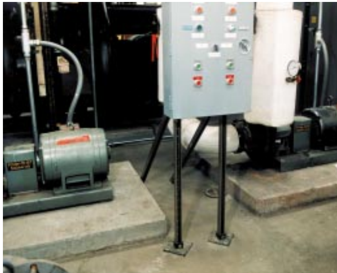
Figure 154: Typical control panel support using angles. Additional angle supports may be required (see below).
