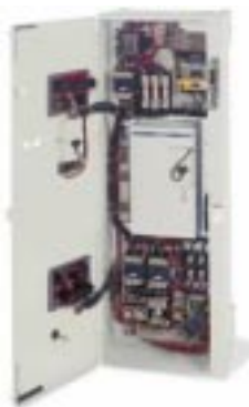
Figure 40: Enclosed motor (wall-mounted).
