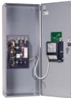
Figure 1: Automatic transfer switch (surface wall-mounted).
