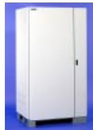
Figure 55: Cabinet battery rack.
