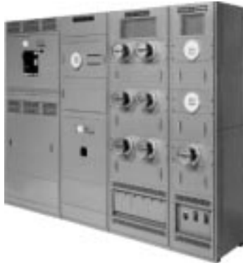
Figure 34: Meter center (floor-mounted).
