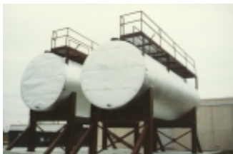
Figure 60: Horizontal tanks including concrete-lined tanks.
