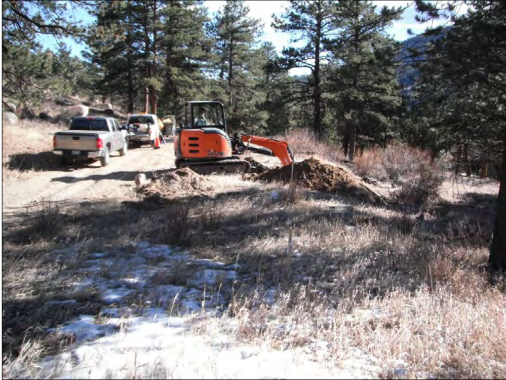
Figure 6. Overview of TP1 and TP3 locations from site 5LR14440, F18, view to the east. Note that TP1 is in foreground and excavation of TP3 is in progress. (Photo roll 20-866, image 6)
